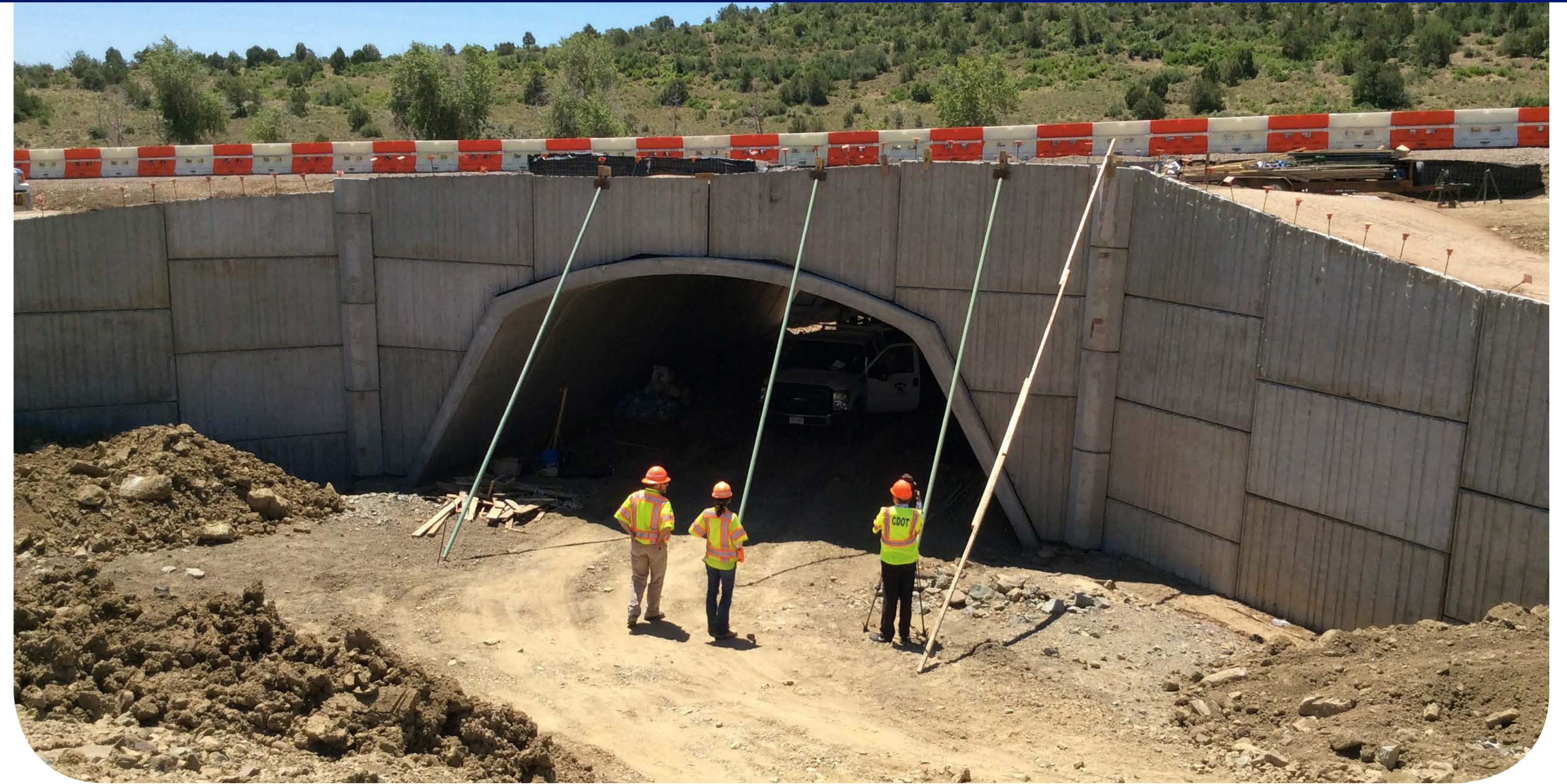
Example of a Wildlife Underpass Crossing that was built at Dry Creek on US 160 in 2016
